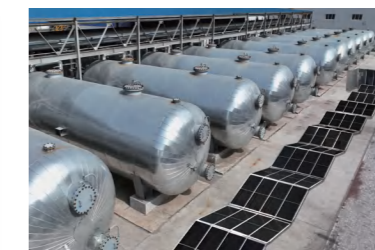
Seawater Treatment Plant
