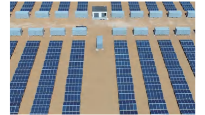
Ground Power Station
