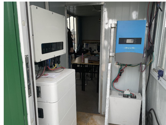
Energy Storage System
